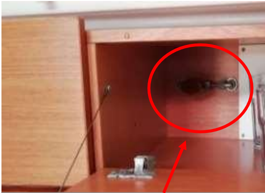
Gas tap ( port side ) , galley.
